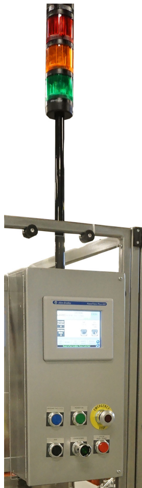
Figure 3-2 - Main Light Stack
